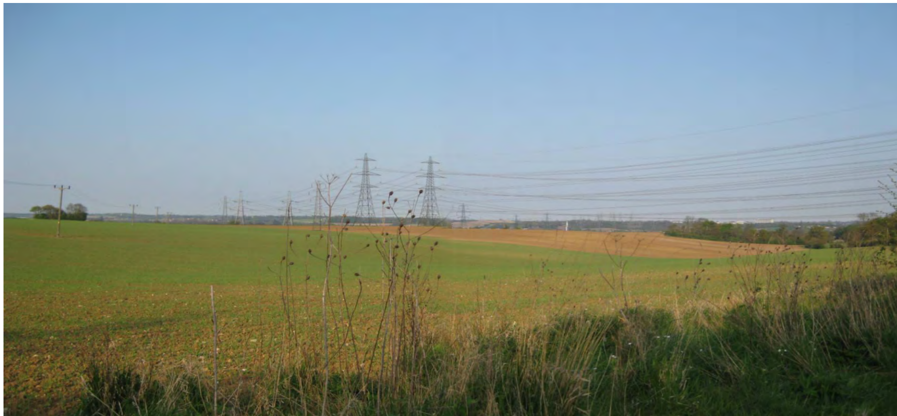
Photographs showing close synchronised paralleling on the existing 400kV parallel overhead lines between Bramford and Sizewell
